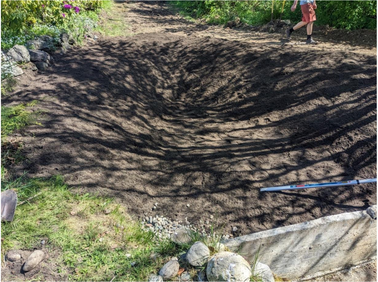
The excavated rain garden site with bioretention soil added in prior to planting. Photo by Bob Simmons.
