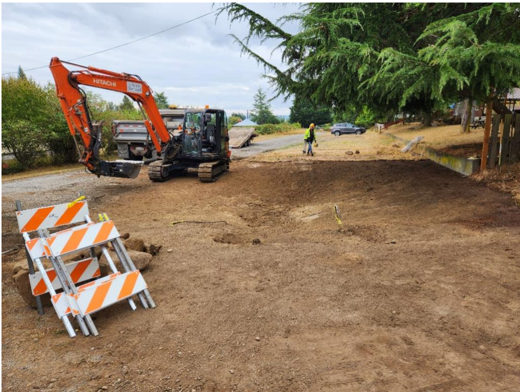
The Swan School site being prepared for the rain garden, with the City of Port Townsend's donated excavation services. Photo by Bob Simmons.
