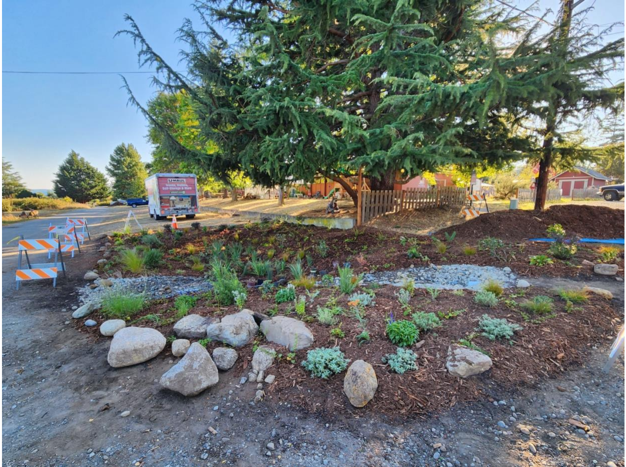
The finished Swan School rain garden after a long day of planting and mulching. Photo by Monica Montgomery.
